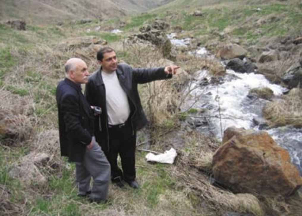
Stepan Ovanessoff (left), administrator of the Mihran and Azniv Essefian Charitable Trust of London, reviewing the renovation of a water holding tank in the mountains high above Aygut with ATP Deputy Director Mher Sadoyan.
